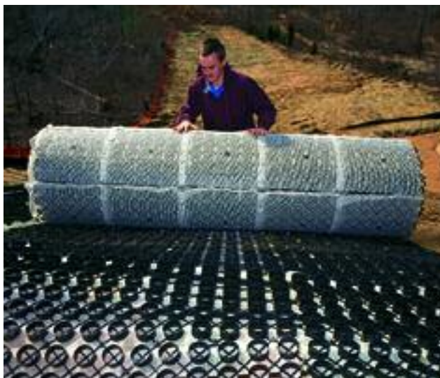
Quick, complete coverage on any slope is easy with large, lightweight rolls in variable widths and lengths to fit site dimensions.
